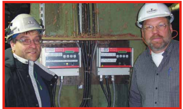
Brady Burke, LP instrument technician (left), and Ed Moar, Electric & Instrumentation Superintendent.
