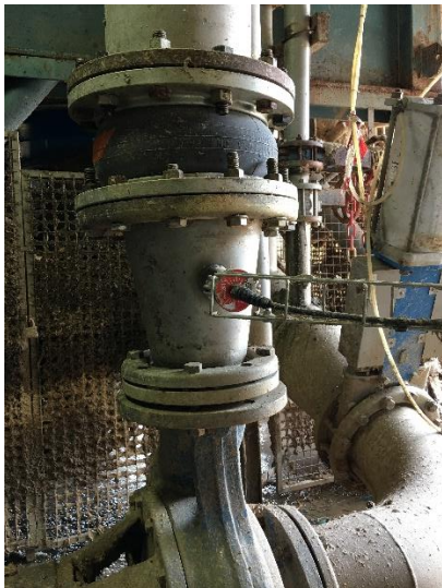
Figure 1: BTG Optical consistency transmitter TCR-2511 installed at the outlet pulper
